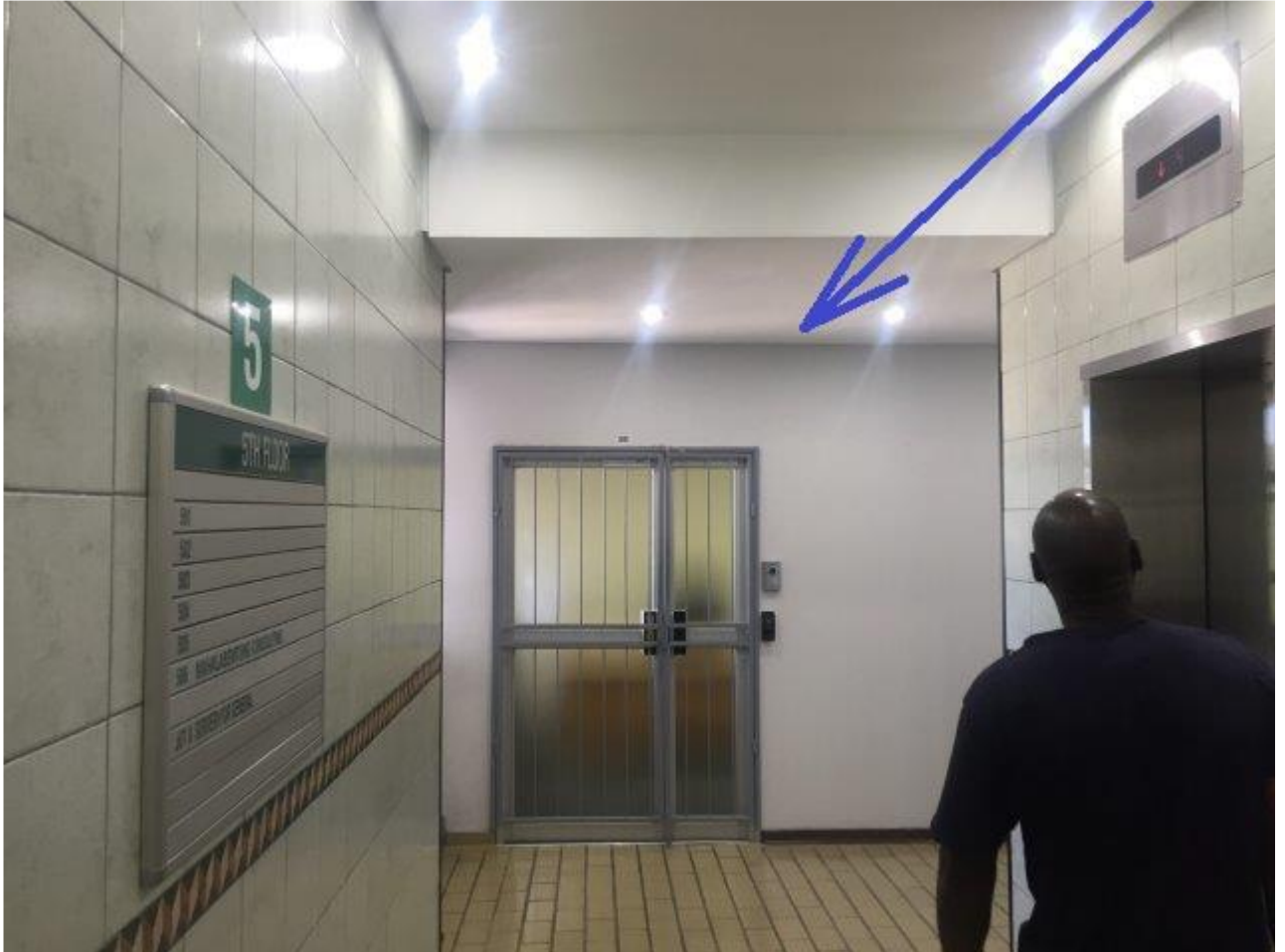
Cable Run (to the office, hidden inside the ceiling))
