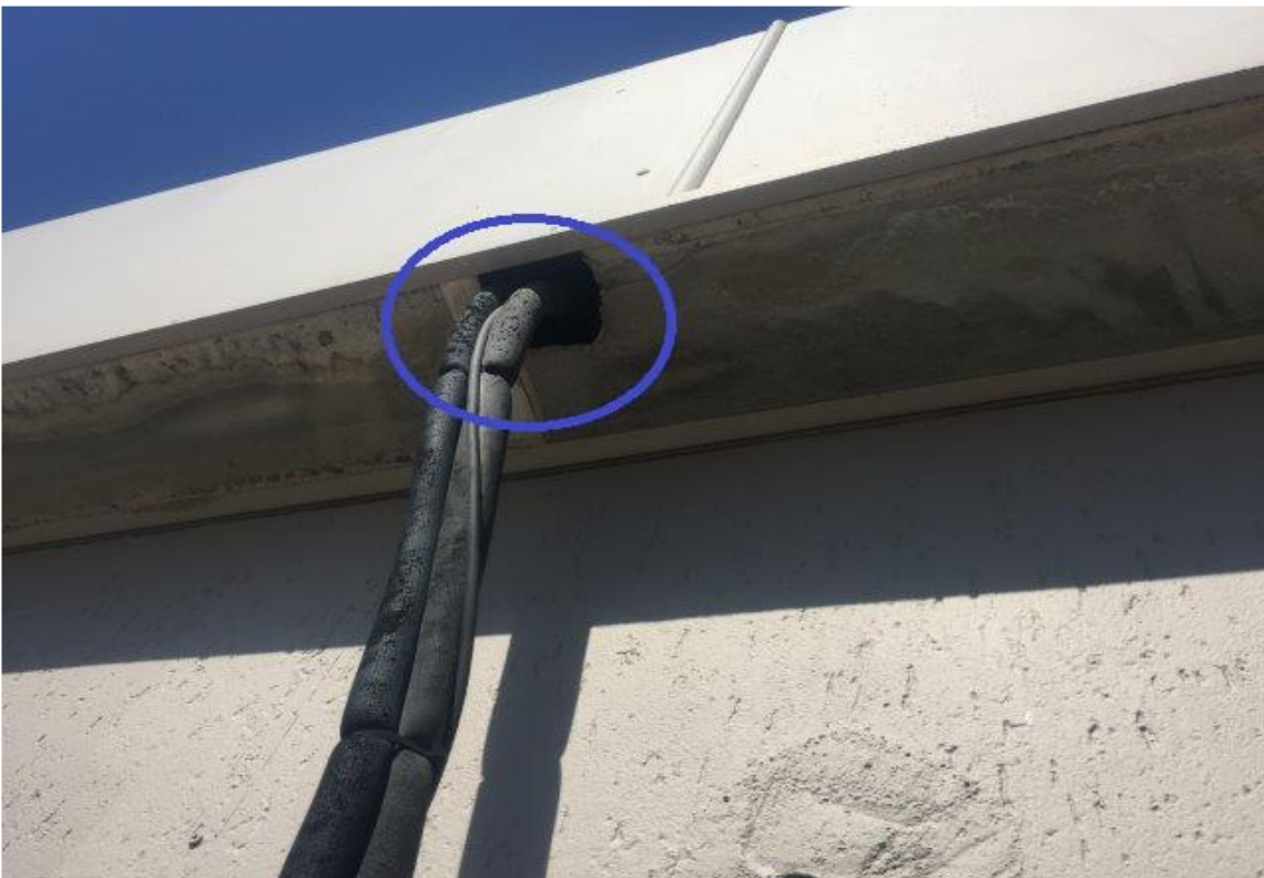
Cable Run (from cable entry, hidden inside the ceiling)
